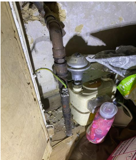
This picture shows incorrect size of cable & Bonded to old disconnected pipe.
